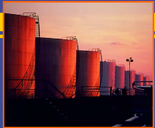
Flammable Liquid Storage
